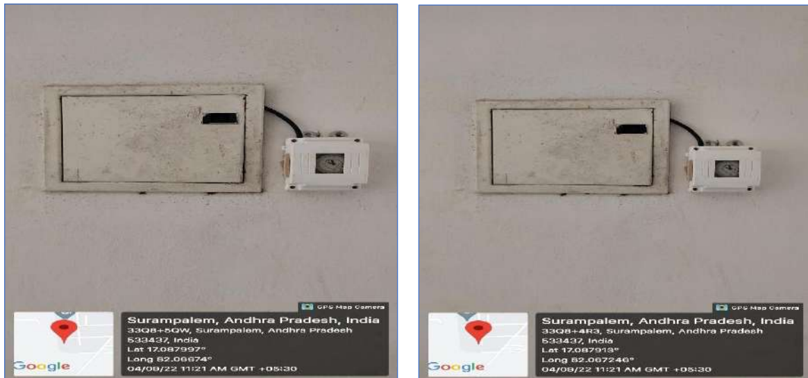
Fig. 4: Sensor-based energy conservation (Location-cotton bhavan)
