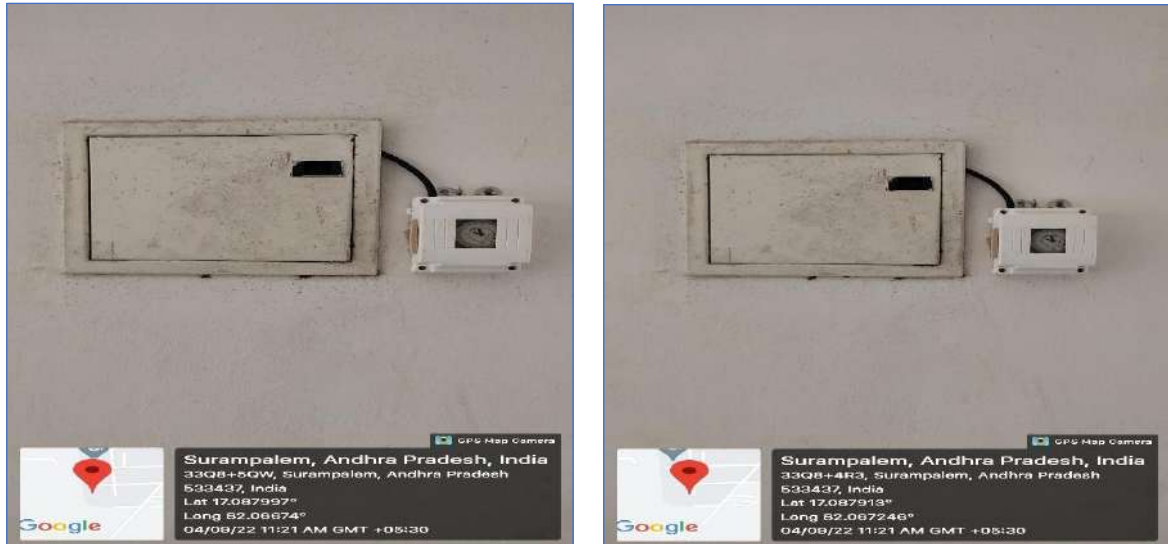
Fig. 4: Sensor-based energy conservation (Location-cotton bhavan)
